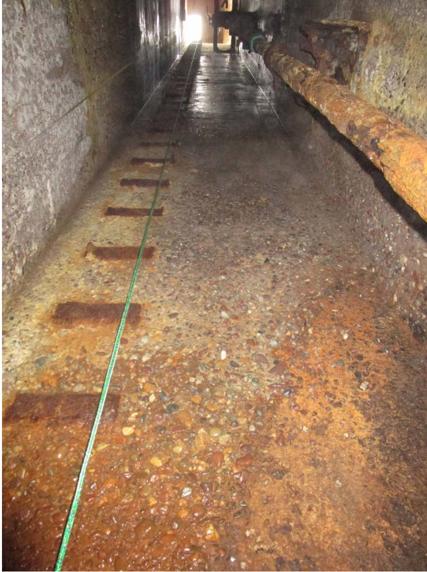
Photo 3 – Concrete surface deterioration and missing ladder rungs on lower portion of tower
