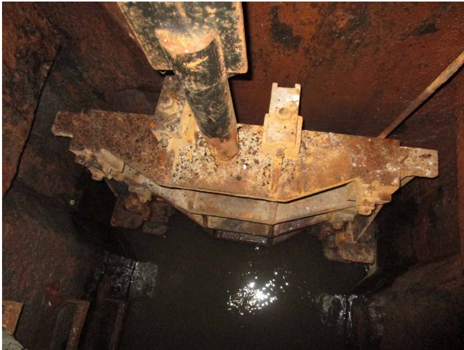
Photo 10 – Existing valve gate
