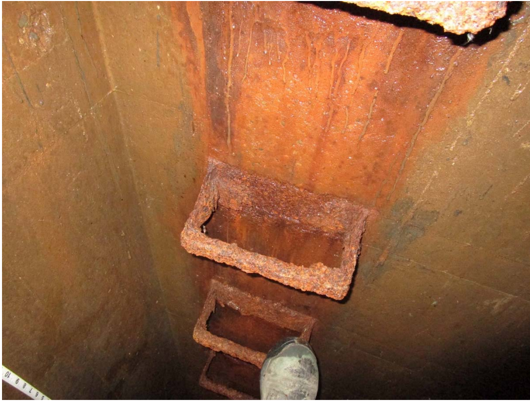
Photo 4 - Typical ladder rung corrosion and section loss
