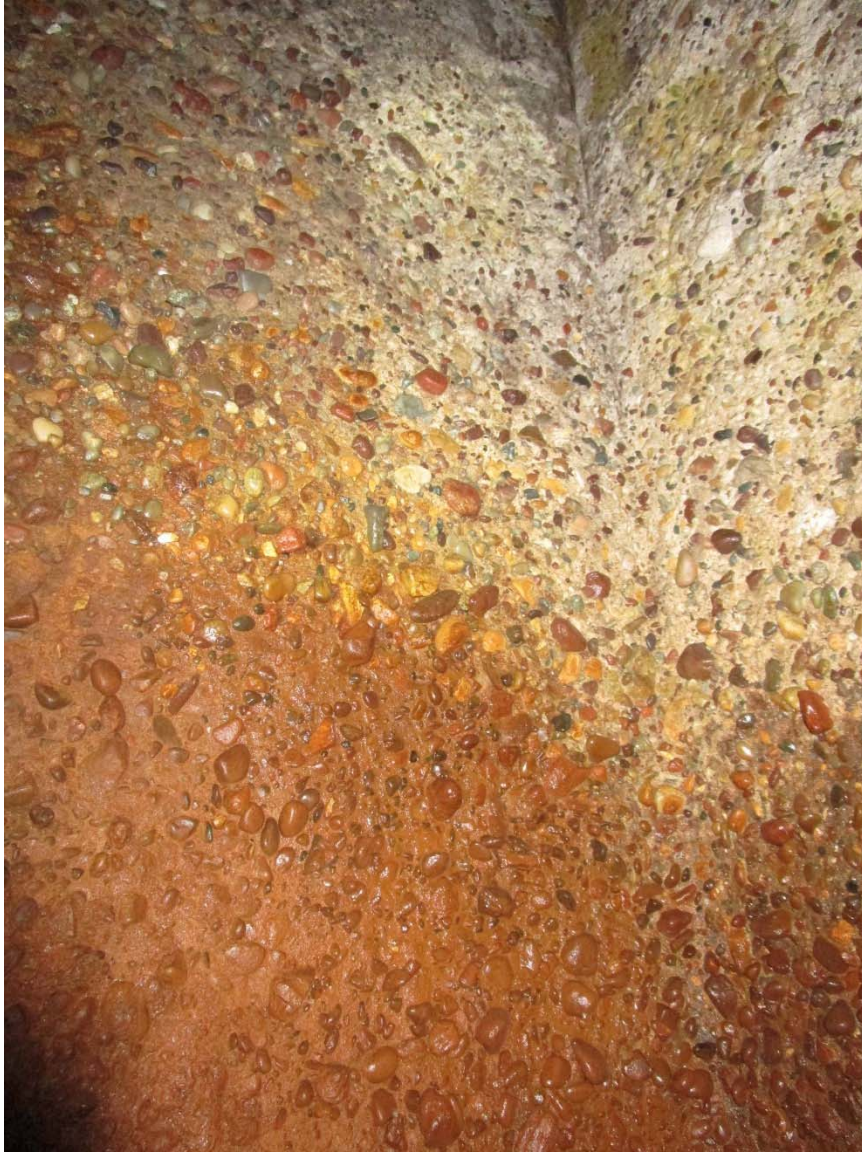
Photo 2 – Typical concrete surface deterioration on lower portion of tower
