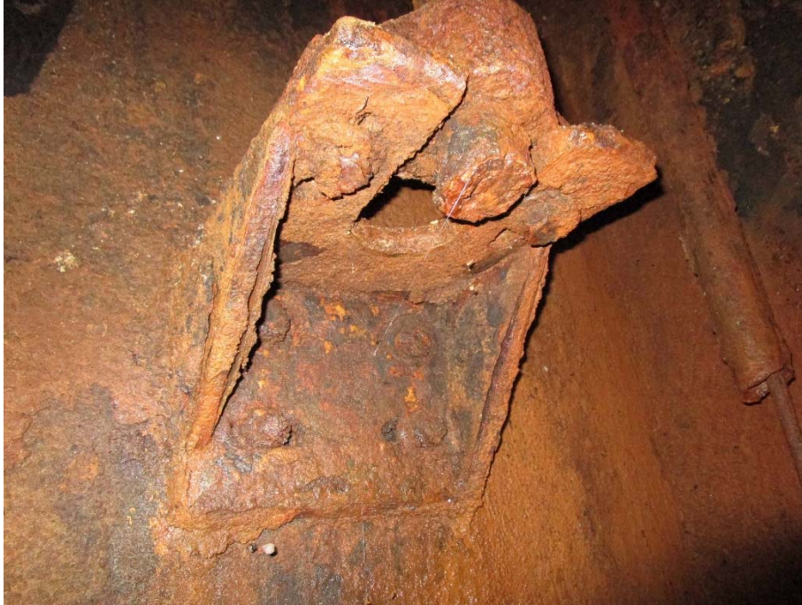
Photo 9 – Typical corrosion and section loss on existing valve equipment
