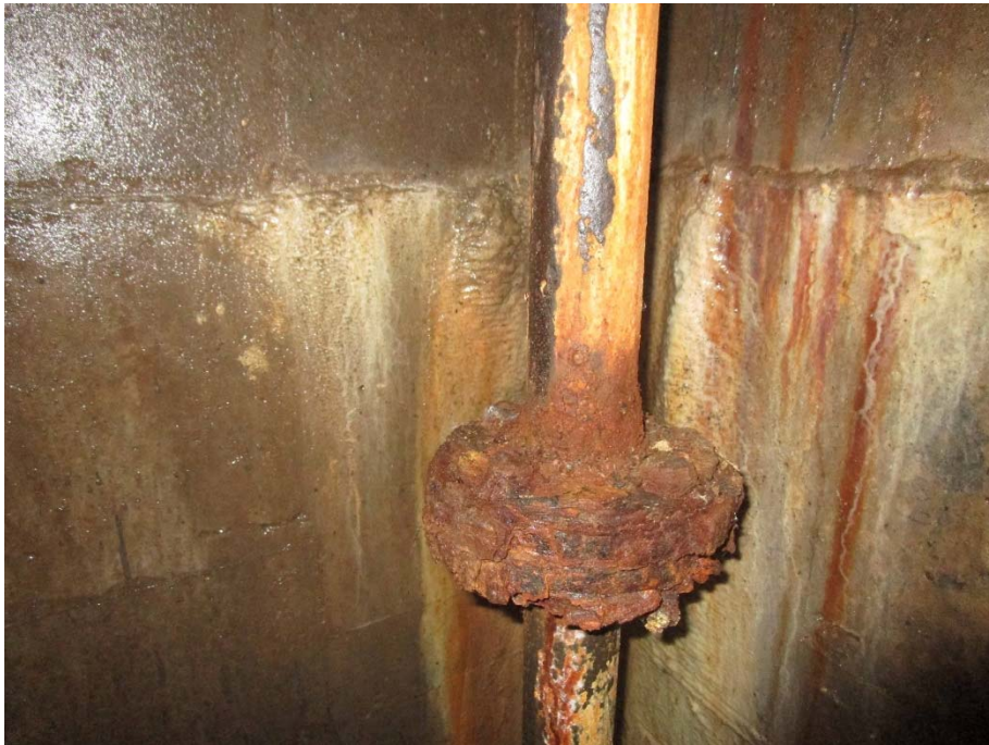
Photo 6 – Efflorescence on north tower wall (31' above base)
