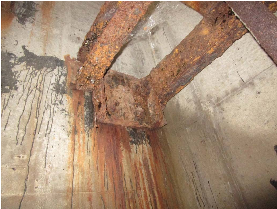
Photo 8 – Typical corrosion and section loss on existing valve equipment
