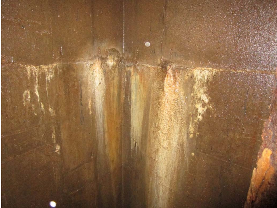
Photo 5 – Efflorescence on north tower wall (31' above base)
