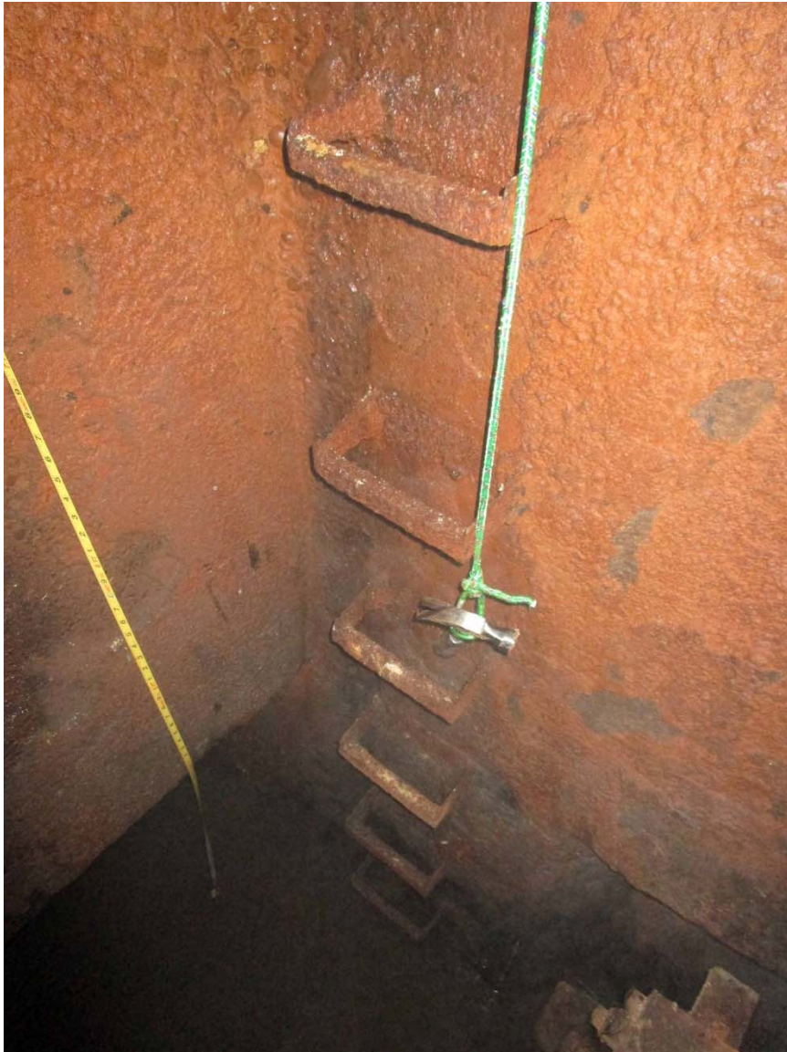
Photo 1 – Typical iron oxide buildup on tower walls near base
